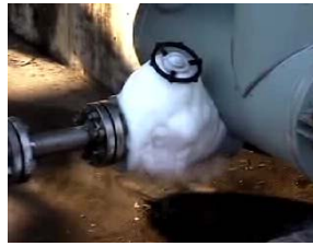
Visible light view of leaking valve
