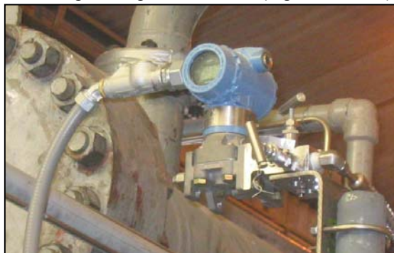
Visible light image of Leak M7 (digital camera)
