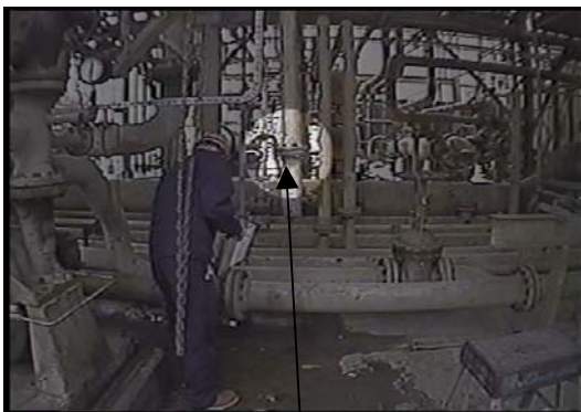
Visible light view of leaking flange
