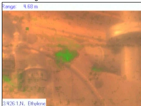
IMSS image of Leak M7
