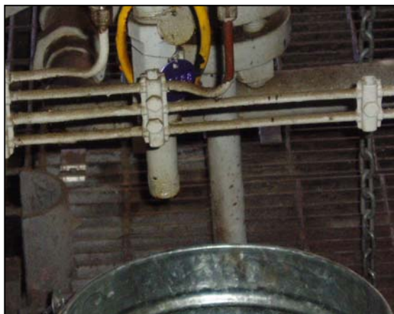
Visible light image of Leak T2 (digital camera)
